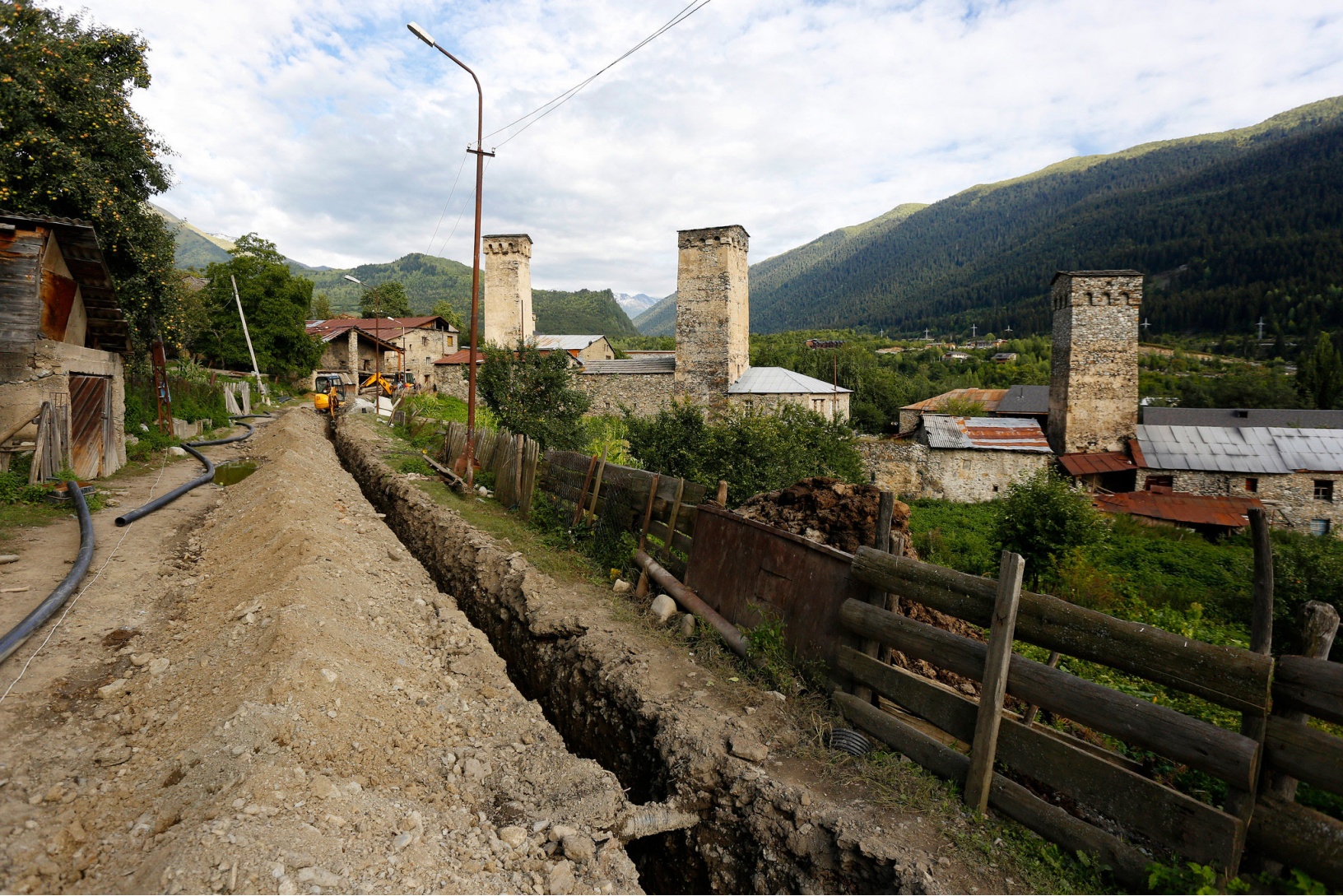
Construction of the Mestia water supply project in Samegrelo-Zemo Svaneti Region, Georgia.
